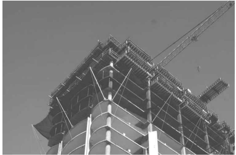
Putting the pieces together on a new luxury hotel going up at Fifth and Howard.
